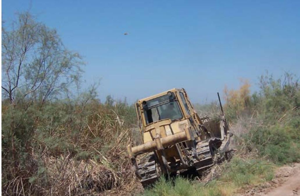
The first step of California Waterfowl's NAWCA enhancement activities this past spring at the Imperial Valley Wildlife Area's Wister Unit was the removal of nearly 10 years of salt cedar and phragmites growth from levees and units.
